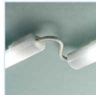
fixture to fixture cable connection
